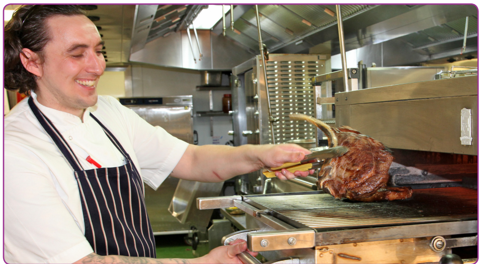
Twin Overfired Broilers in service
